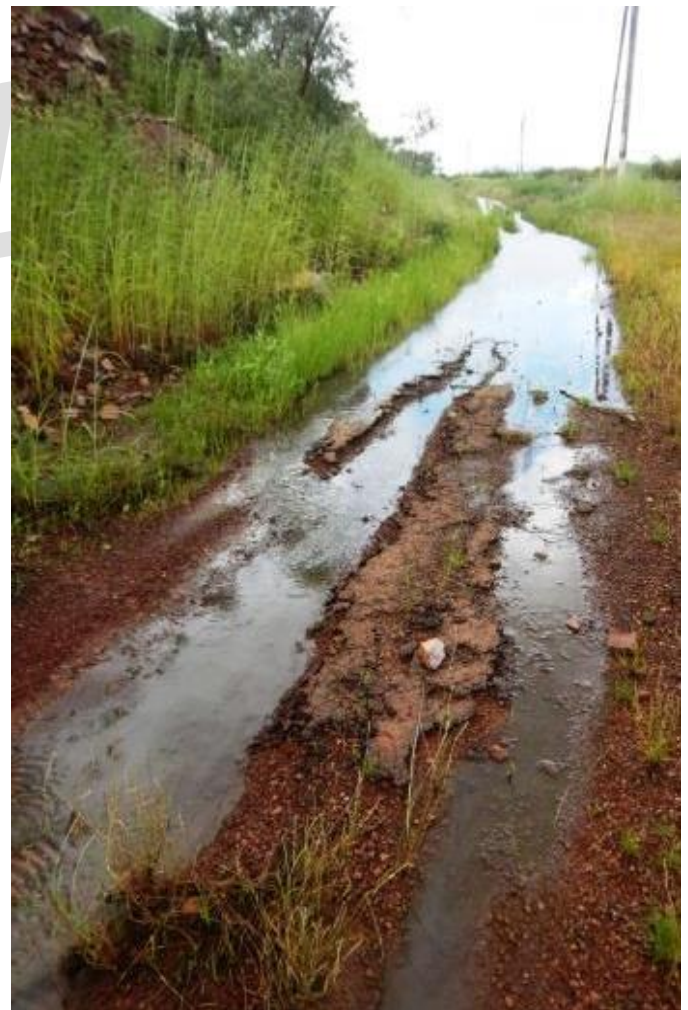
Image 19: Extensive Damage to Wyndham Port Path
