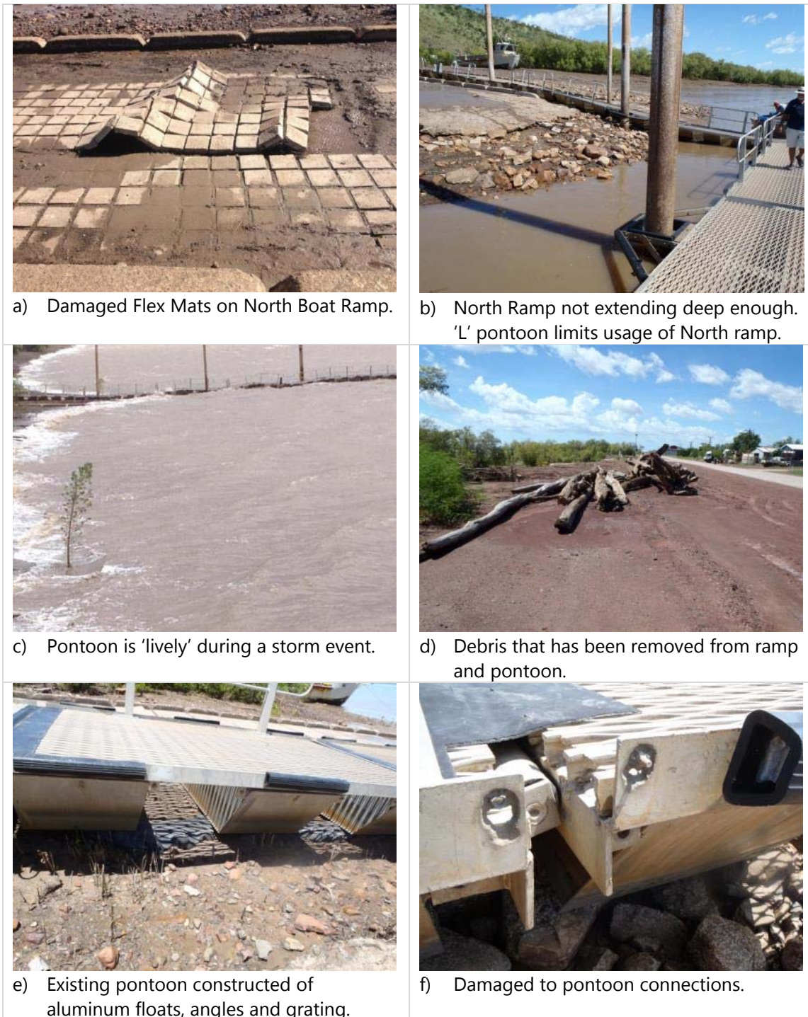
Figure 4-1 Issues with Existing Boat Launching Facility
