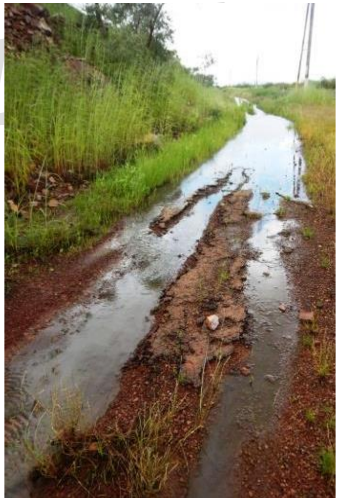
Image 19: Extensive Damage to Wyndham Port Path
