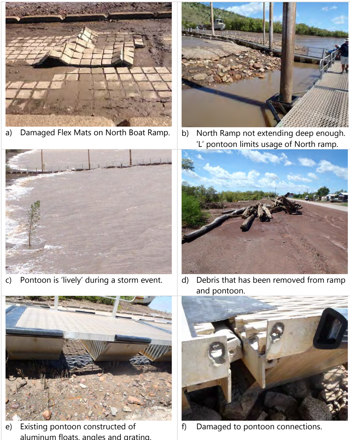
Figure 4-1 Issues with Existing Boat Launching Facility
